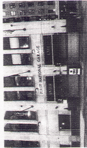
Figure 4: Existing unreviewed sign above garage with horizontally oriented letters intersecting with plaster.
