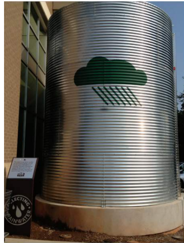
Cistern with informational signage, Raleigh, NC
