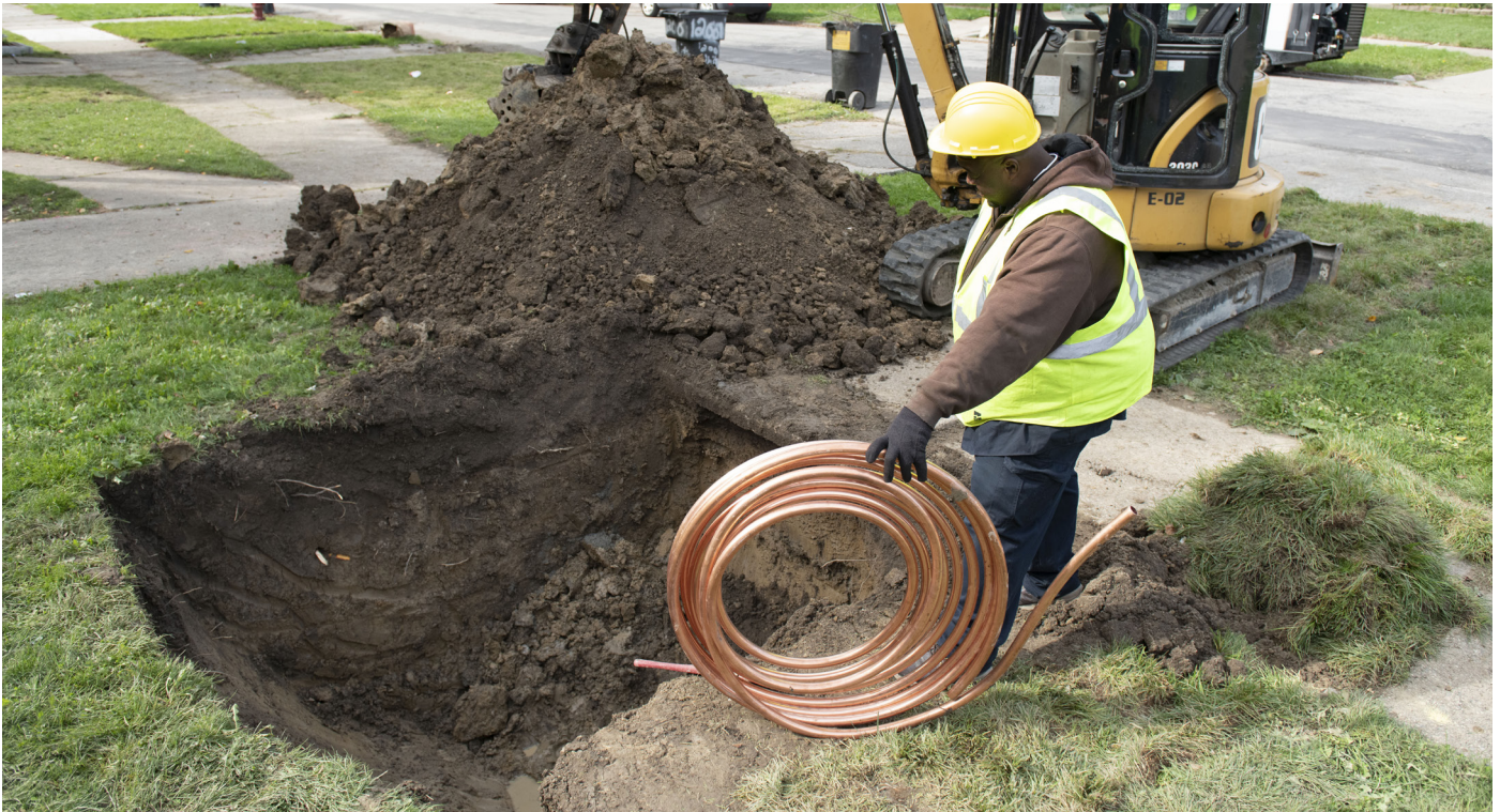
In 2018, DWSD began replacing lead service lines with copper, with owner/occupant permission, while on the same street replacing the water main.
