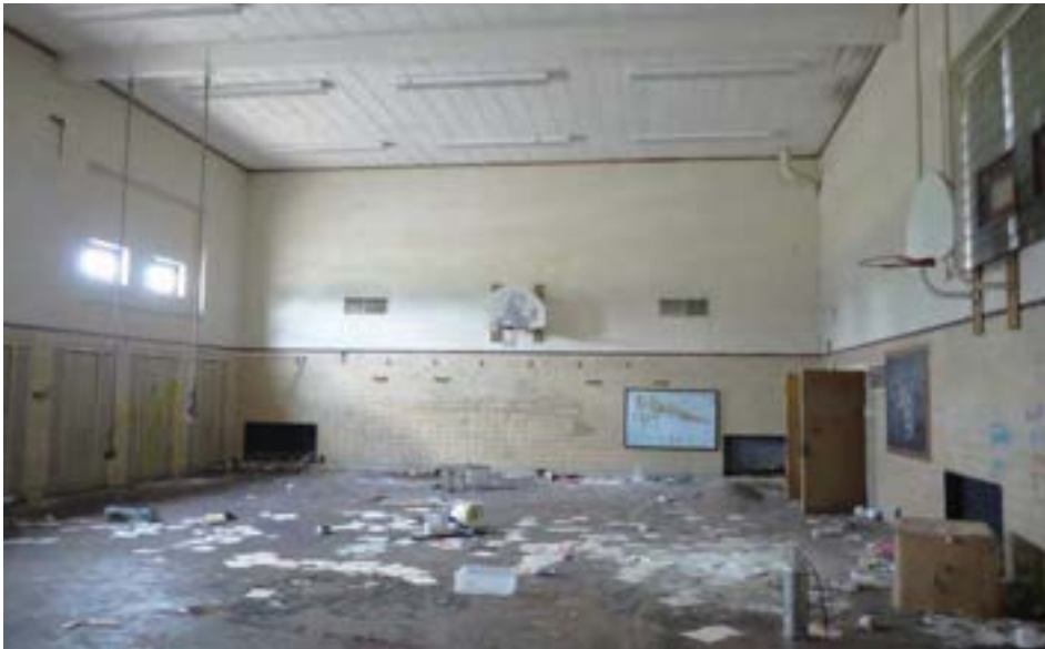
Gym/Cafeteria. Original glass block windows have been mostly covered (brick over exterior) and replaced with small lites
