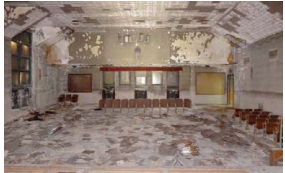
The auditorium has been damaged by smoke and the seating has mostly been stolen. The southwest school entrance can be closed off so that the vestibule only serves the rear of the auditorium.
