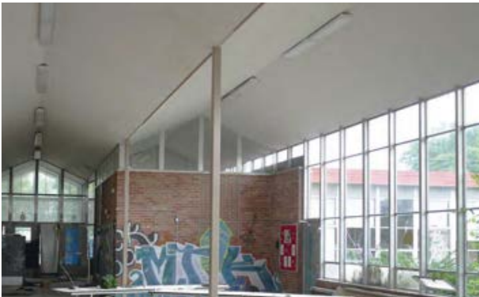
Glass box entrance lobby. Large single-glazed window wall provides ample natural light and creates an airy feel; however, it may also be susceptible to solar gain in summer and heat loss in winter.
