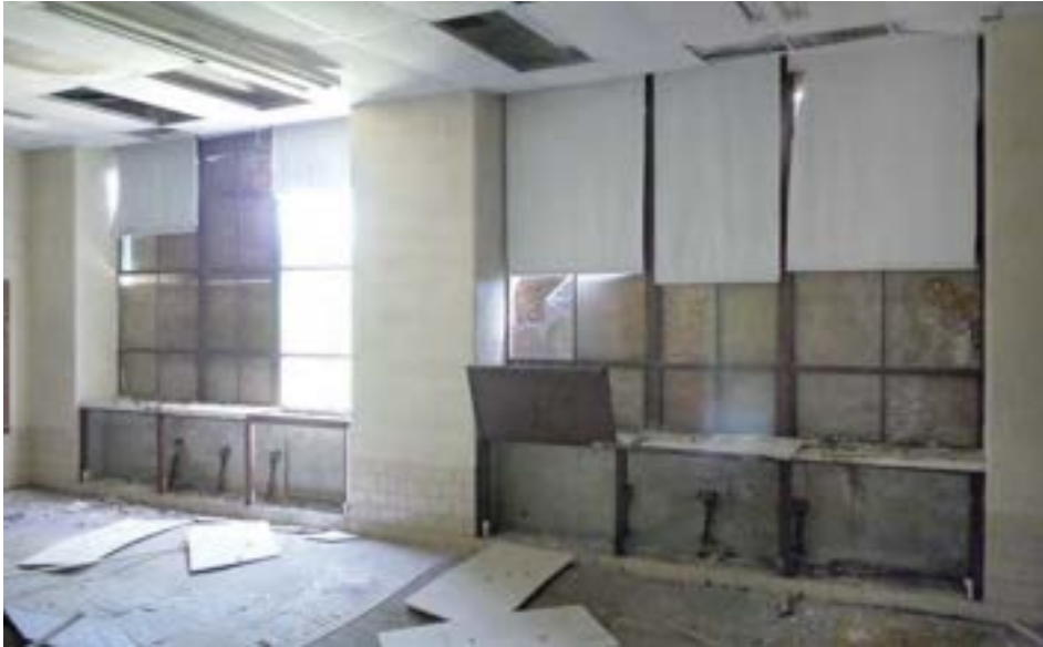
Operable steel-framed windows in the historic school building are largely intact, but in need of repair. Classroom construction is simple concrete block.
