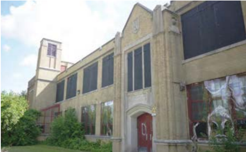
West (main) elevation, showing newer addition. Original 1921 unit is visible behind tower in background.
