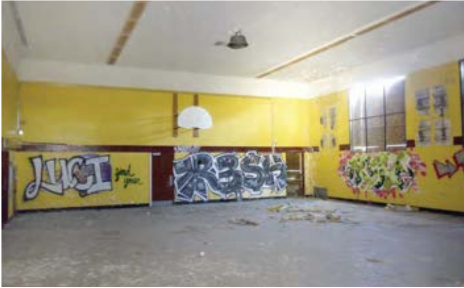
The northwest gym is a simple brick box with high windows and 18' ceilings. There is an identical space on the southwest corner of the building that was formerly a gym converted into high-ceilinged classrooms.
