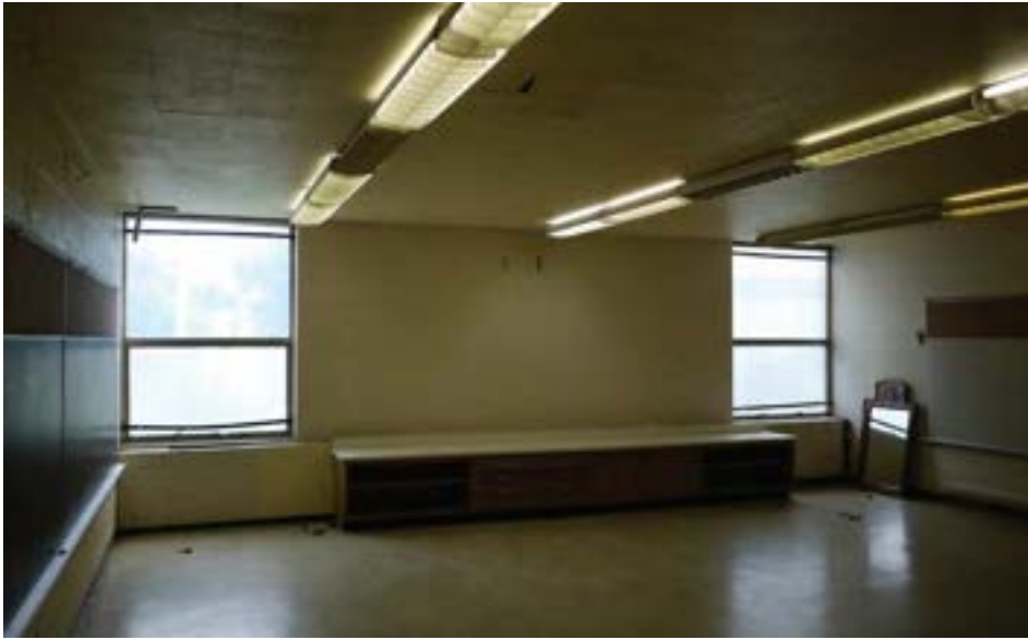
Typical classrooms feature two corner windows facing either north or south. Finishes are simple: painted concrete, acoustic tile ceiling, and vinyl tile floors. Other than minor water staining, there is very little visible distress.
