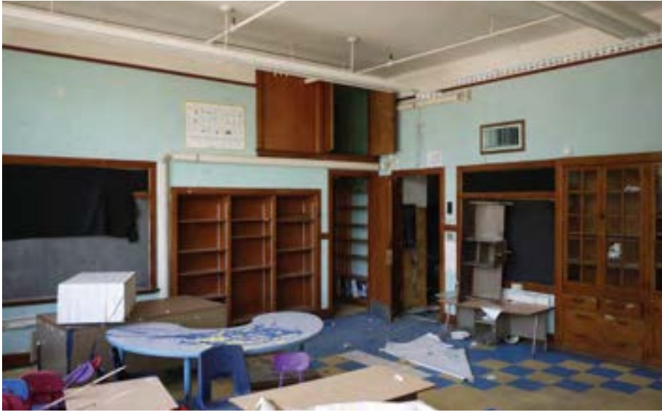
This classroom, perhaps a former art room, features a large amount of original built-in wood cabinetry and shelving, including a large high cupboard area.
