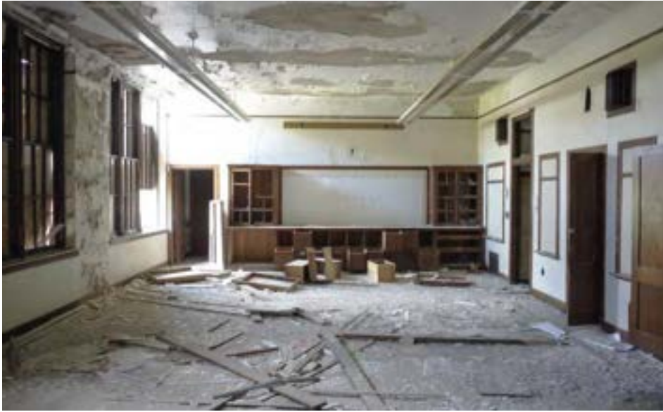
A specialty classroom in the original wing featuring a large wood built-in storage unit.
