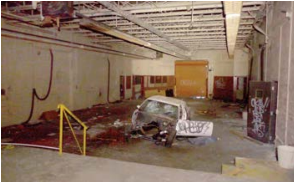
The automotive shop was formerly an open courtyard with a ramp to the rear parking lot. A steel joist roof and garage door were added to close off the space.
