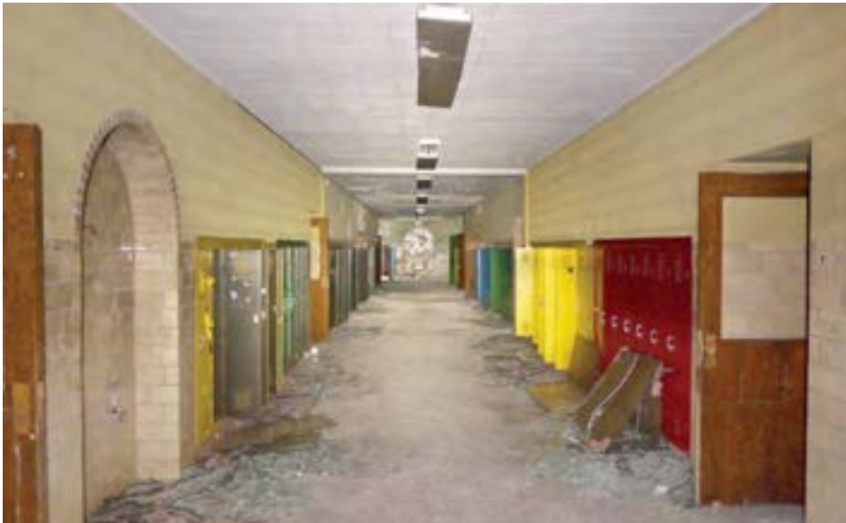
Classroom corridor in excellent condition. CMU and glazed block wall construction with intact lockers and arched drinking fountain alcoves.
