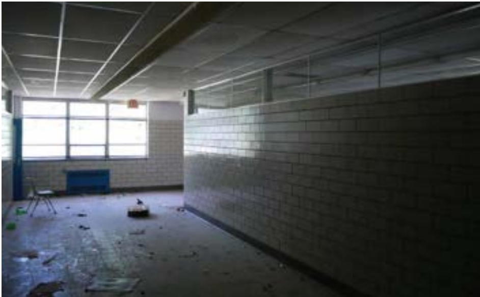
A corridor in the 1961 unit showing measures to allow natural light. Finishes are in good condition.
