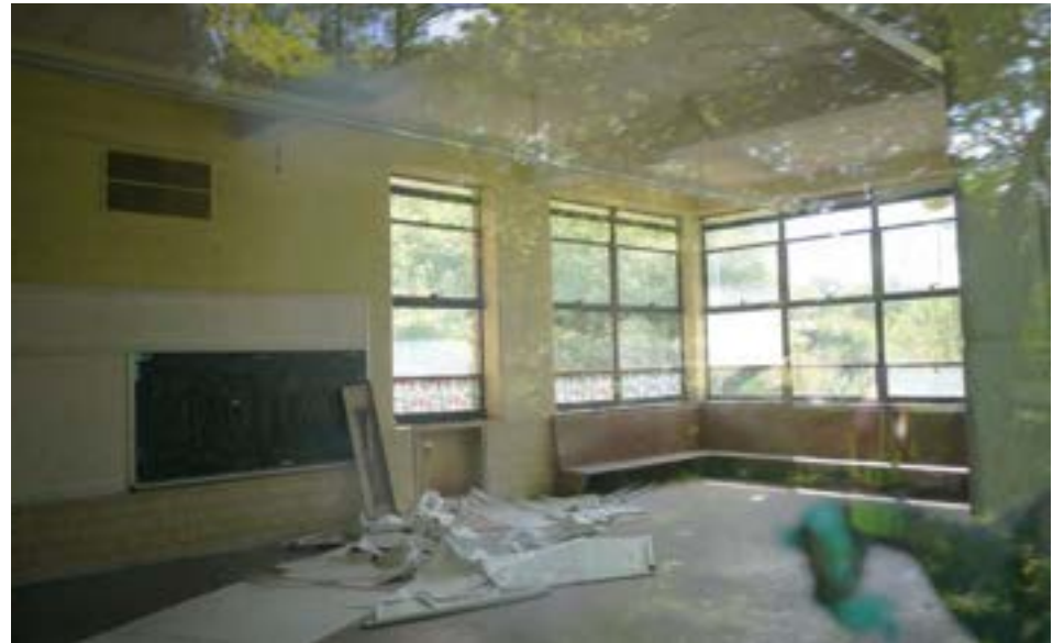
The 1948 kindergarten includes a rectangular bay window and wooden bench. Like other classrooms spaces viewed from the outside, this room appeared to be in very good condition, with few signs of distress.
