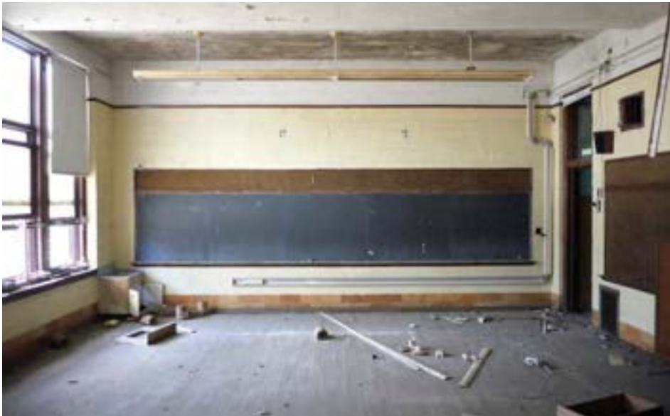
Typical classroom with CMU walls. Wood finishes are in excellent condition and contemporary aluminum windows are intact. Note mold/water staining on ceiling.
