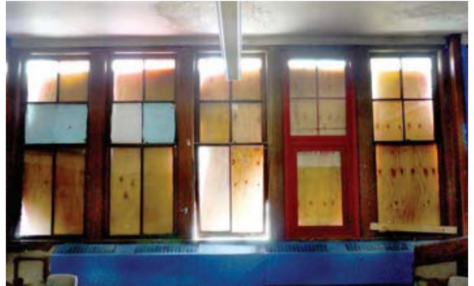
Classroom windows are typically intact and in repairable condition. Modern emergency escape windows have been added in each classroom, though the majority of the windows are original wood frames.
