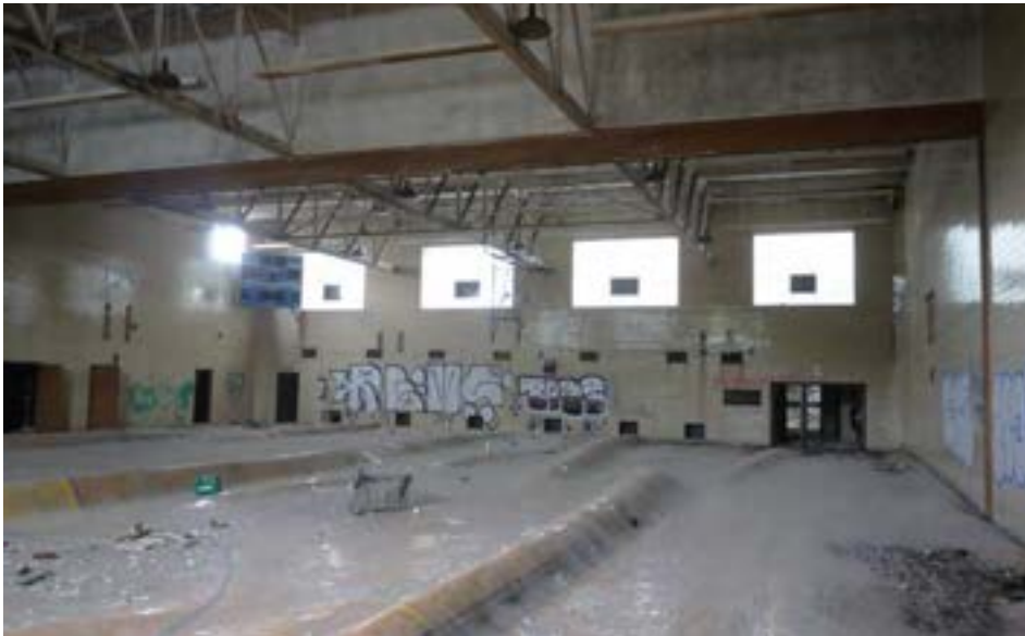
The 1955 gymnasium is large, featuring a full-size basketball court. The gym can be divided into two halves using a sliding wood partition. The wood floor is heavily bowed, and there is prominent step-cracking visible on the masonry wall where the gym joins the original school building.
