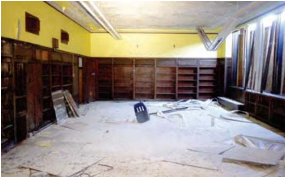
The library is slightly larger than a typical classroom and features built-in wood shelving around the perimeter. Finishes are in fair condition.
