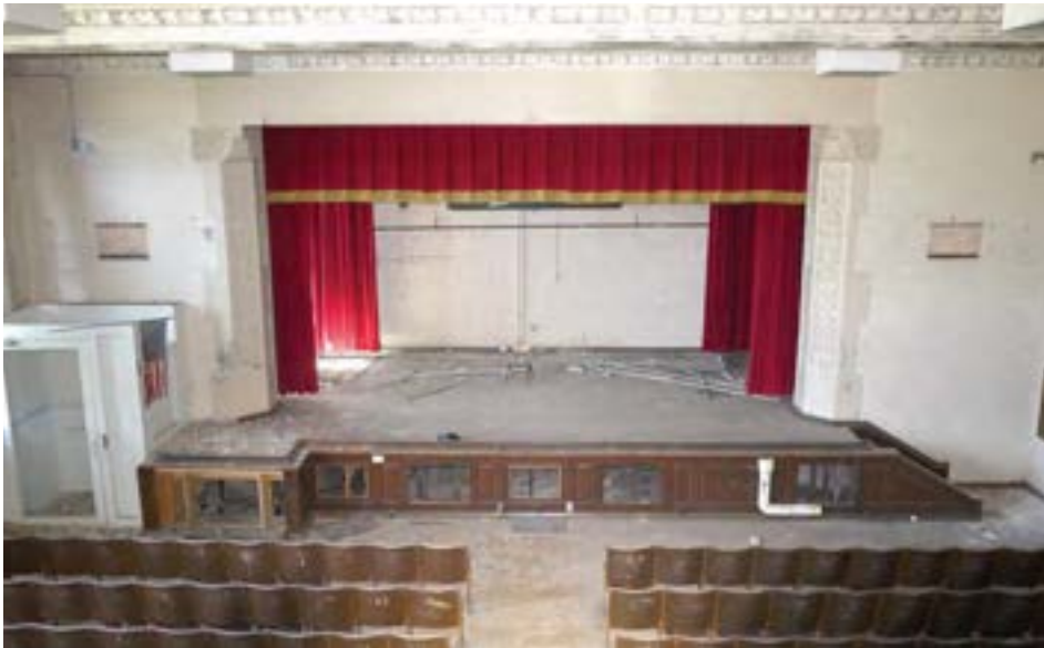
Auditorium viewed from mezzanine projector room. The space is constructed of CMU, but with cast-concrete and plaster decorative elements. A modern wheelchair lift has been added to the left of the stage.
