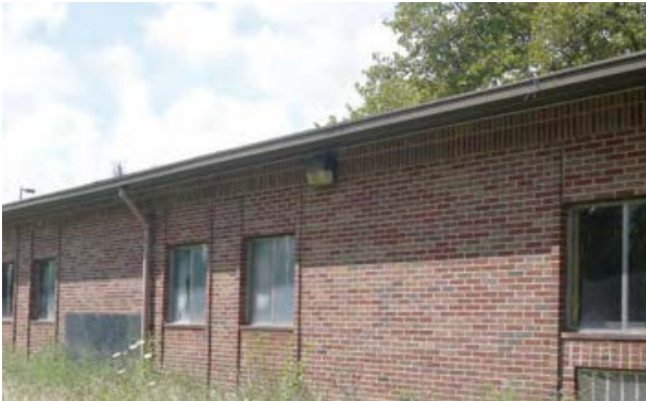
A single-story classroom addition was attached to the southeast corner of the building in an unknown year. The steel-frame, gable-roofed, double-loaded structure appears similar to other 1970s era additions observed in this study.
