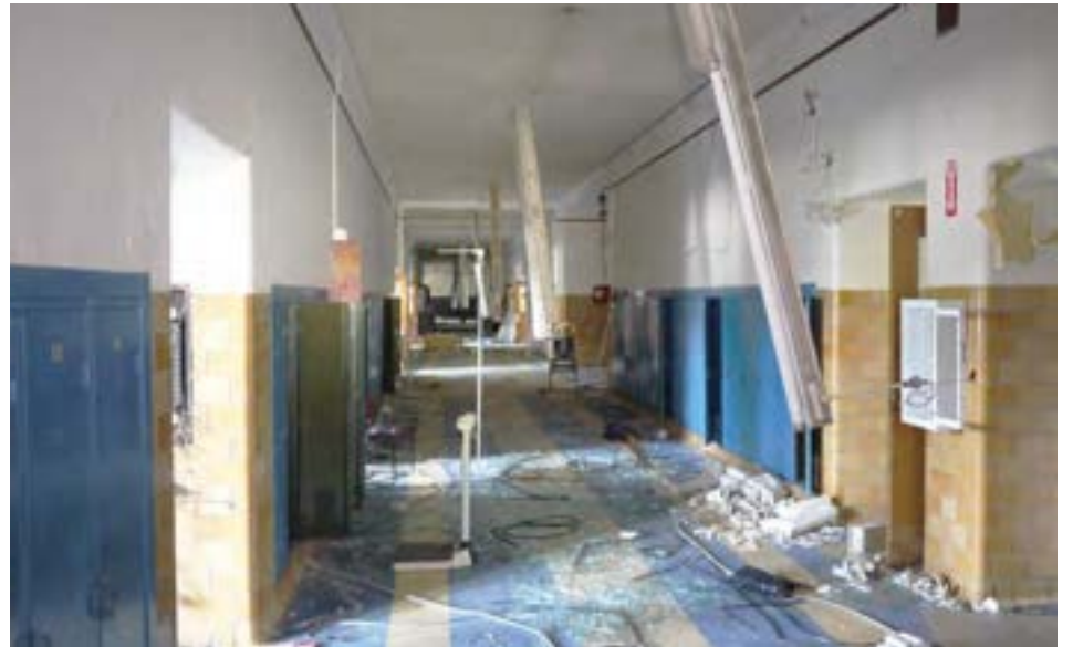
North first floor hallway, showing glazed block and plaster finishes in good condition. Other hallways exhibit some water damage and scragging damage.
