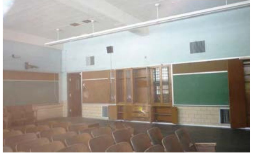
A classroom in the 1955 unit appears to be in very good condition, with few signs of distress to the finishes. This room appears to be storing the wood seating from the auditorium.
