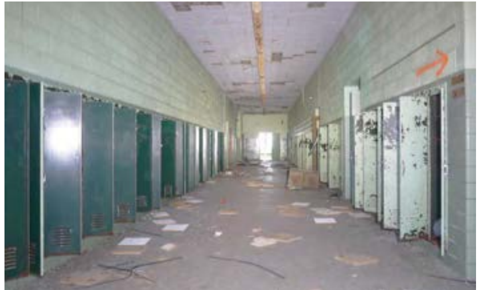
The double-loaded first floor corridor, featuring simple, durable finishes in good condition. Walls are painted CMU with glazed block; floors are terrazzo.
