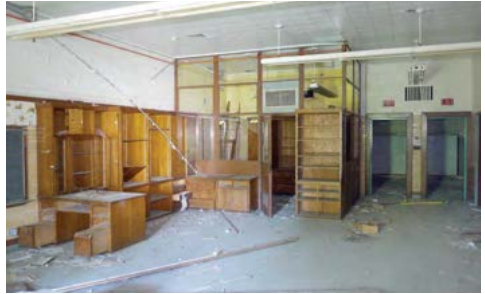
The "general arts" room on the second floor is a large room occupying the center of the building. It includes built-in wood casework and work tables that are in repairable condition. In this newer portion of the building, finishes are CMU and glazed brick.
