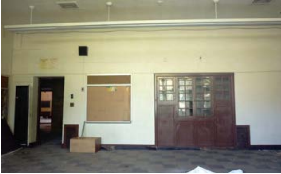
A classroom in the 1930s unit appears to be in very good condition, with painted concrete walls, vinyl tile floors, and acoustic tile ceilings with very few signs of distress.
