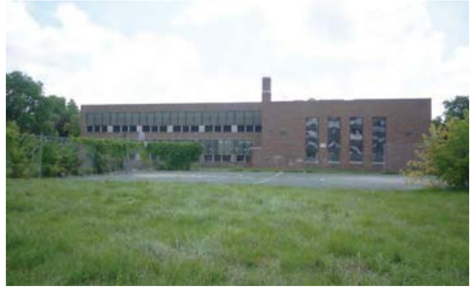
North elevation showing 1942 auditorium (left) and 1955 classroom addition (right). Playfield and basketball court are visible in foreground.
