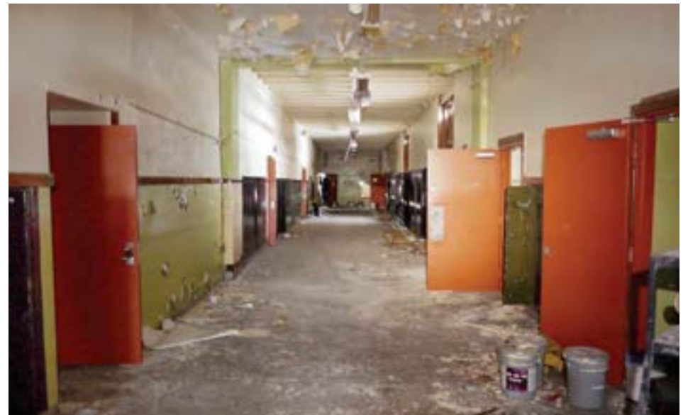
The main south corridor on the first floor is oversized at 14' wide and 14' high. This view shows the transition from 1928 plaster finish (foreground) to 1948 concrete finishes (background)
