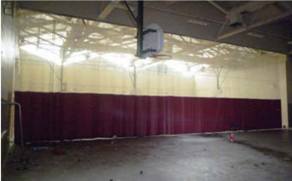
Full-size gym with divider curtain closed. The gym receives diffuse natural light from its large diamond-shaped fiberglass panels.
