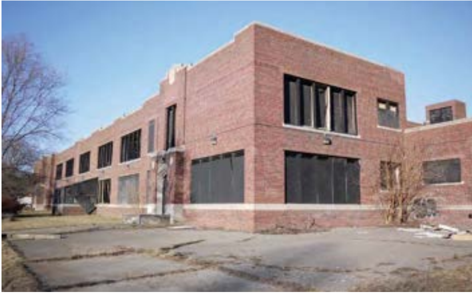
Southwest wing viewed from Meyers Road. The southern addition was part of a large expansion in 1930-1931, but care was taken to match the style of the original building.
