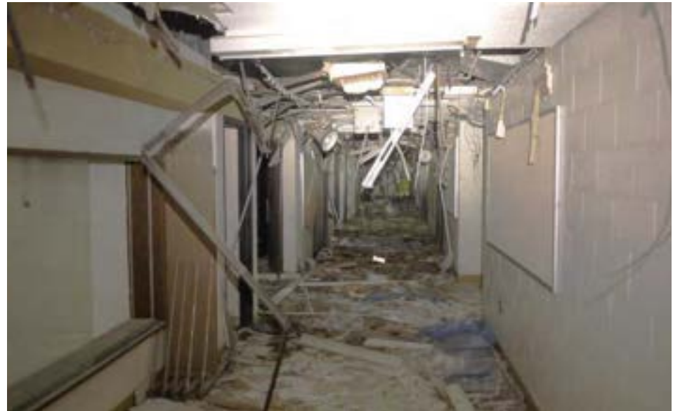
The main hallway's drop ceiling has been torn apart and scrapped. Other finishes are durable and could be cleaned/repared.
