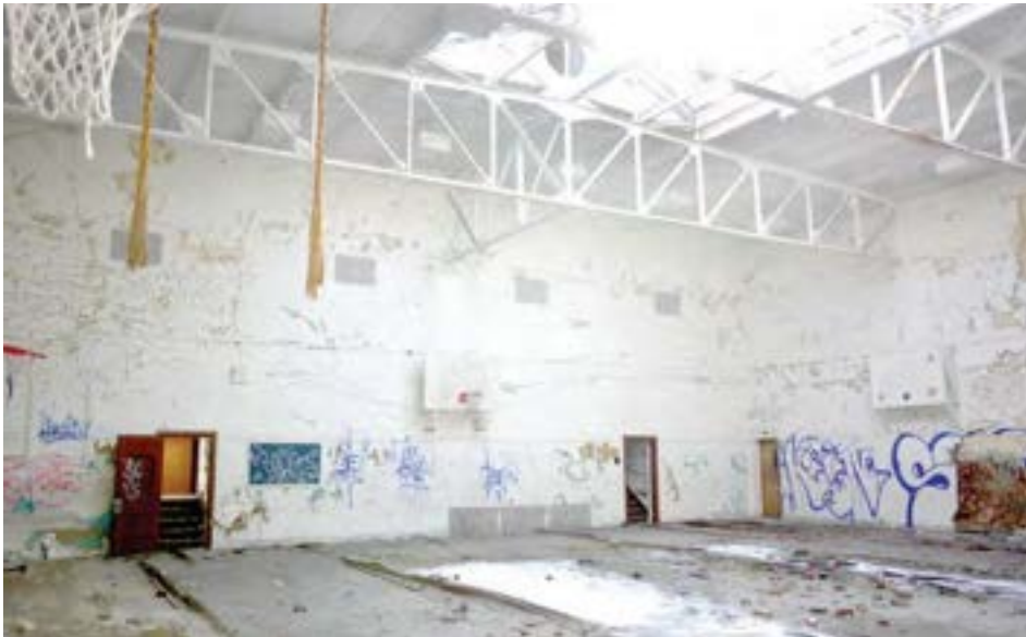
The gymnasium is located in the center of the building and is lit naturally by a single large skylight. The effect is a soaring, airy space that is unique among elementary school gyms.
