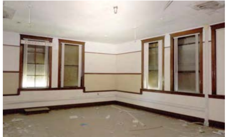
Classrooms in the 1914 unit are in generally good condition, with many original plaster and wood finishes intact and in repairable condition. All classrooms in this building are located in corners, allowing for windows on two exposures.
