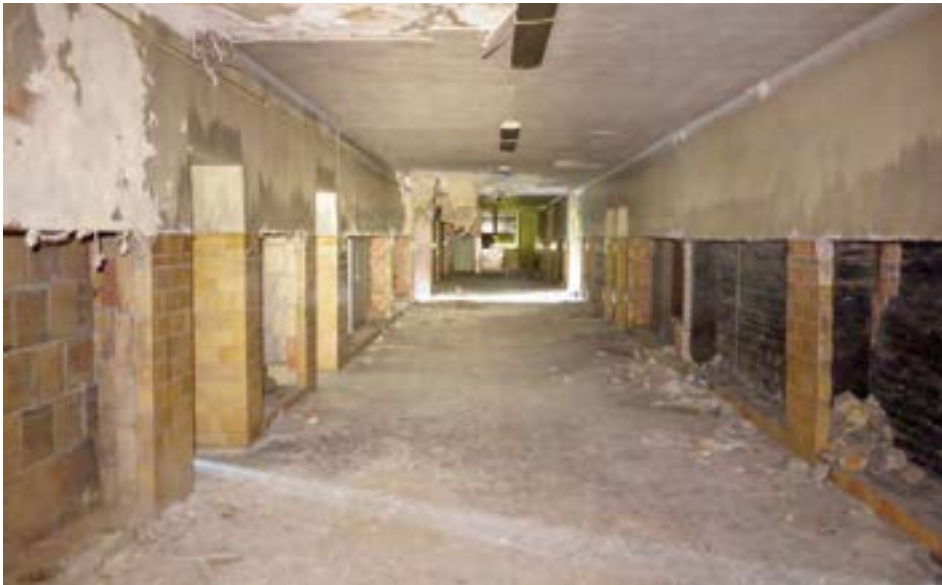
The wide second floor main corridor is finished with plaster, buff glazed blocks, and terrazzo floors. Lockers, plumbing, and ductwork have been scrapped, but the overall condition is fair.
