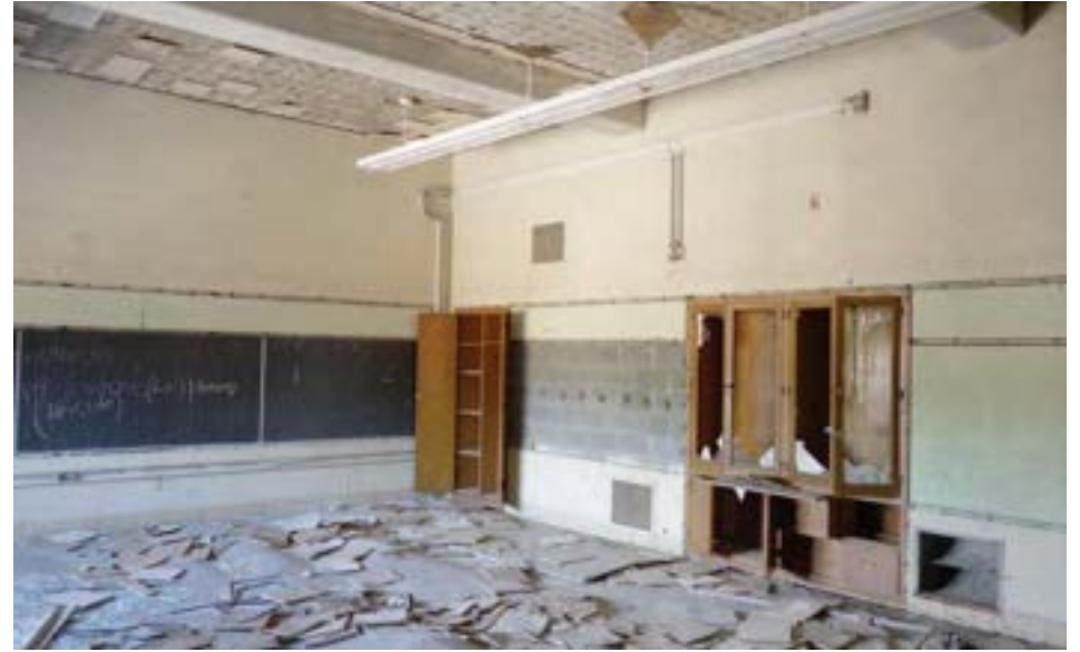
Typical classrooms in the 1946 and 1951 additions are plain, with CMU walls, exposed concrete beams, and extra-high ceilings.
