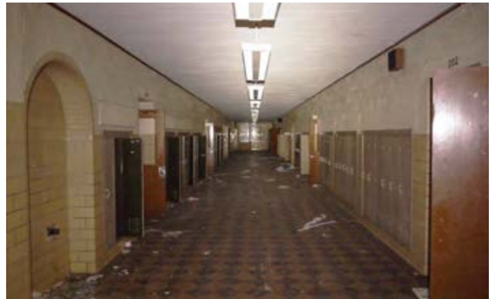
Typical corridor in good condition. Corridor finishes are painted CMU and glazed block, with vinyl tile floors.
