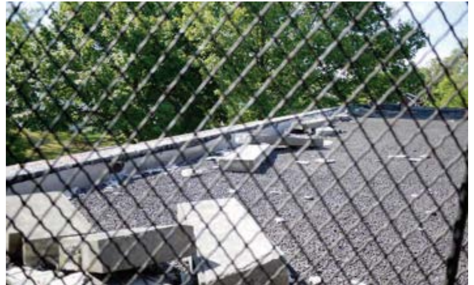
Coping stones pushed onto the roof by scappers; metal flashing has been taken, leaving wall construction exposed.
