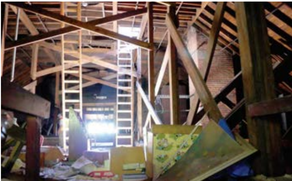
The 1914 building features a tall wood-framed attic beneath the hip roof. The attic is unfinished and was used for textbook storage before the school closed. It could be converted into an interesting space.
