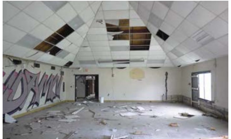
Multipurpose room, featuring a large pyramid roof, similar to the smaller classroom spaces. This space served as gym, cafeteria, and auditorium. There are two exits to Salsinger Playfield.
