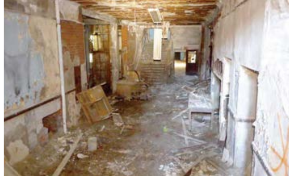
The 1922 unit is heavily water damaged due to a deteriorated roof. Interior walls are primarily gypsum block and plaster, and not in salvageable condition. However, the concrete frame structure may still be serviceable.
