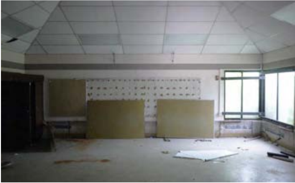
A typical classroom, featuring the school's trademark pyramid roof and aluminum-framed corner windows.
