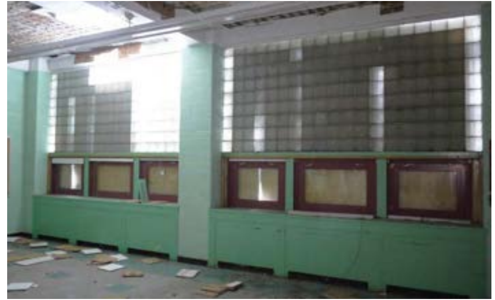
Typical 1950 classroom in good condition. Glass block windows have been retained, but original steel frame lites below have been replaced with more efficient aluminum windows.
