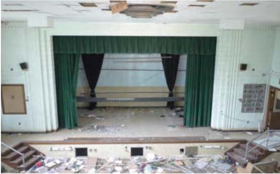
The stage area viewed from the auditorium's balcony seating area. The auditorium is constructed of CMU, but includes decorative geometric elements that echo the exterior design.
