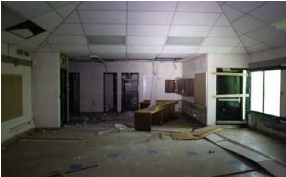
North specialty classroom featuring an extension area with restrooms, storage, and sink area. This classroom is the only one that features its own exit, which leads to Salsinger Park.
