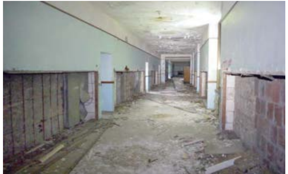
The long western corridor, as seen from the 1921 south addition, looking towards the original 1915 main corridor.
