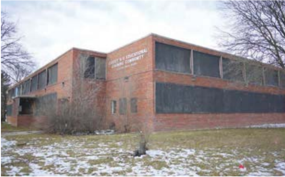
1954 south and east wings viewed from Cambridge and Gilchrist Streets. Long ribbon windows—once filled with glass block—run along the length of these elevations.
