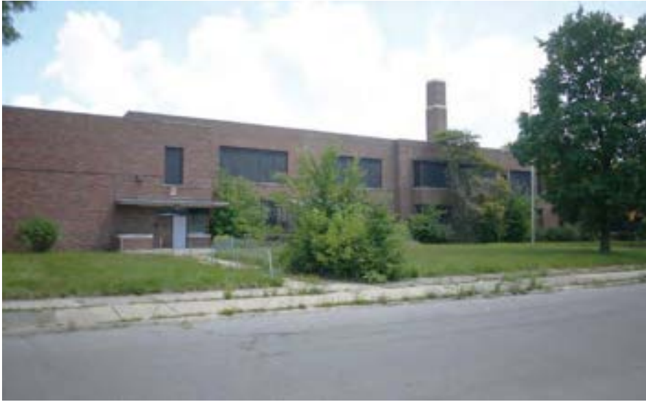
Main West elevation showing 1930 and 1942 additions. The 1942 auditorium and entrance are visible to the left of the frame.
