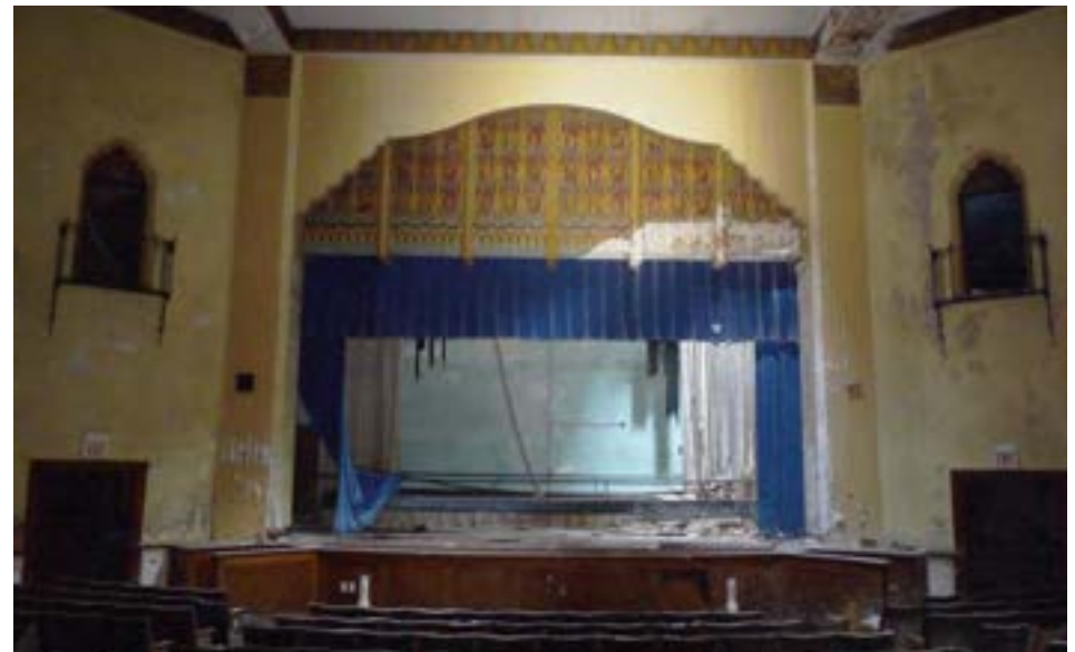
The large auditorium features a unique Spanish/Moorish motif with rich colors and geometric patterns. The stage and balcony area are water damaged and have open holes in the roof caused by scraping activity.
