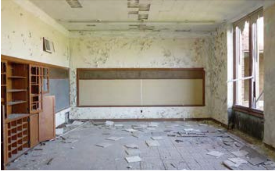
A second floor classroom in the older half of the building, finished with plaster. Classrooms in the 1948 wing are painted CMU. Windows and radiators have been scrapped throughout, but this room is otherwise in relatively good condition.
