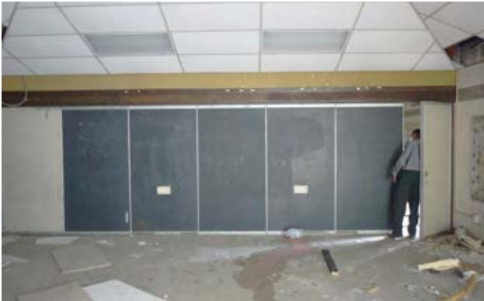
Classrooms at the south end of the building are separated by movable partition walls, which allows for the creation of larger spaces.
