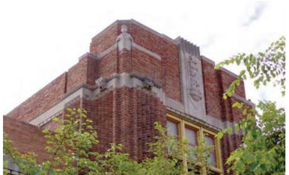
Cast stone details on the parapet above an entrance, including gargoyles, sunflower, and student with book.
