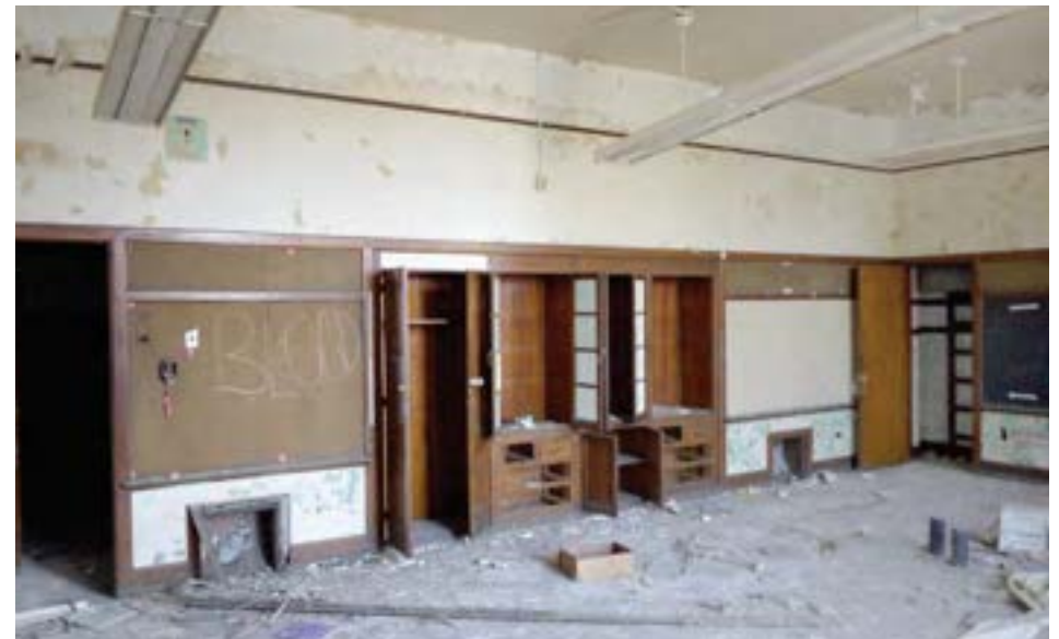
Typical built-in cabinetry in classrooms. This example is in good condition. A closet with wooden ladder leading to a roof hatch is visible in the far right corner.
