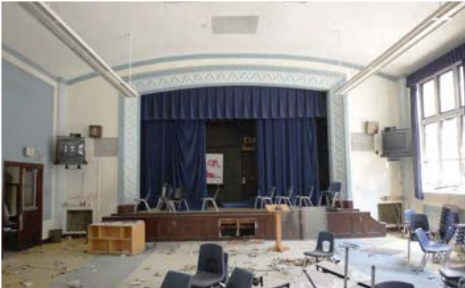
The main auditorium is a flat-floored box with a barrel-vaulted ceiling and large windows facing the central light-well. The plastered finishes are in excellent condition and appear to have been restored and painted recently.
