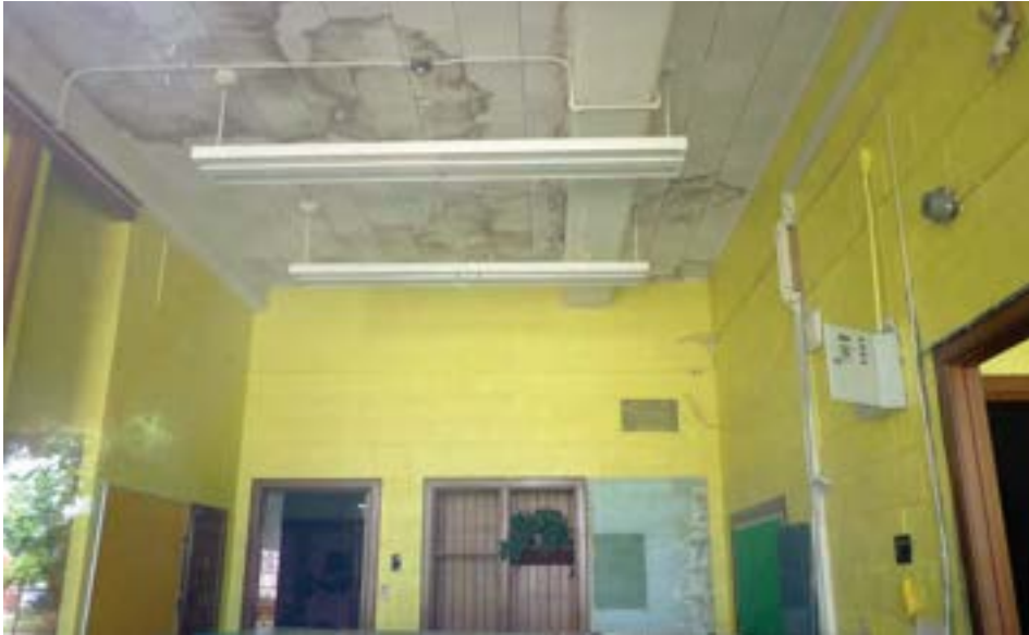
Office with water staining (observed from outside)
