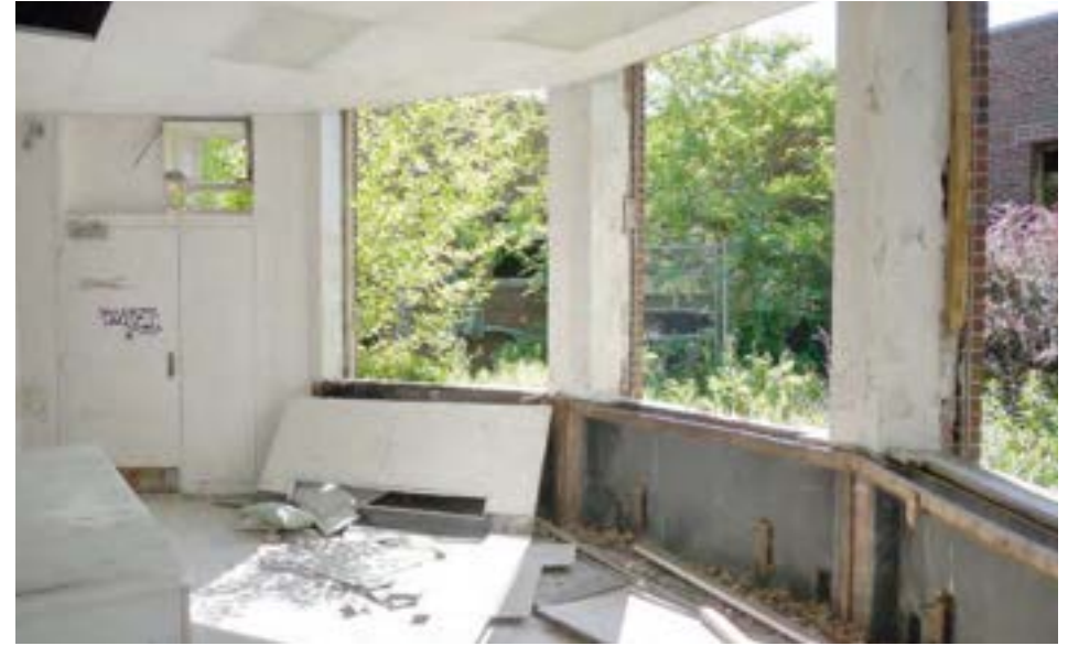
Inside the former kindergarten bay window, looking into one of the two remaining interior courtyards.
