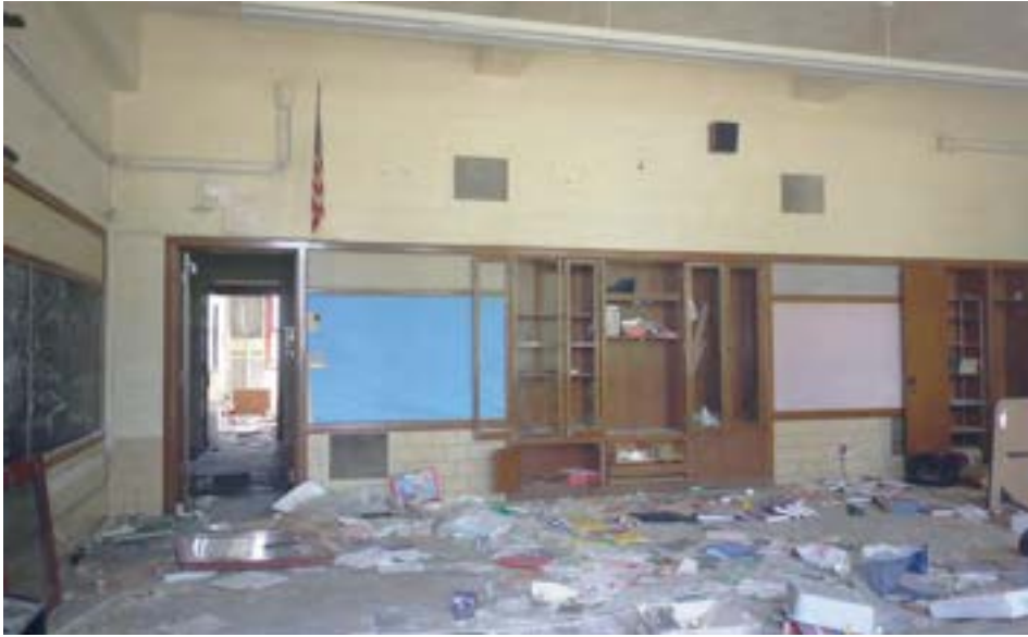
Classroom in addition, showing concrete frame and CMU walls (observed from outside)
