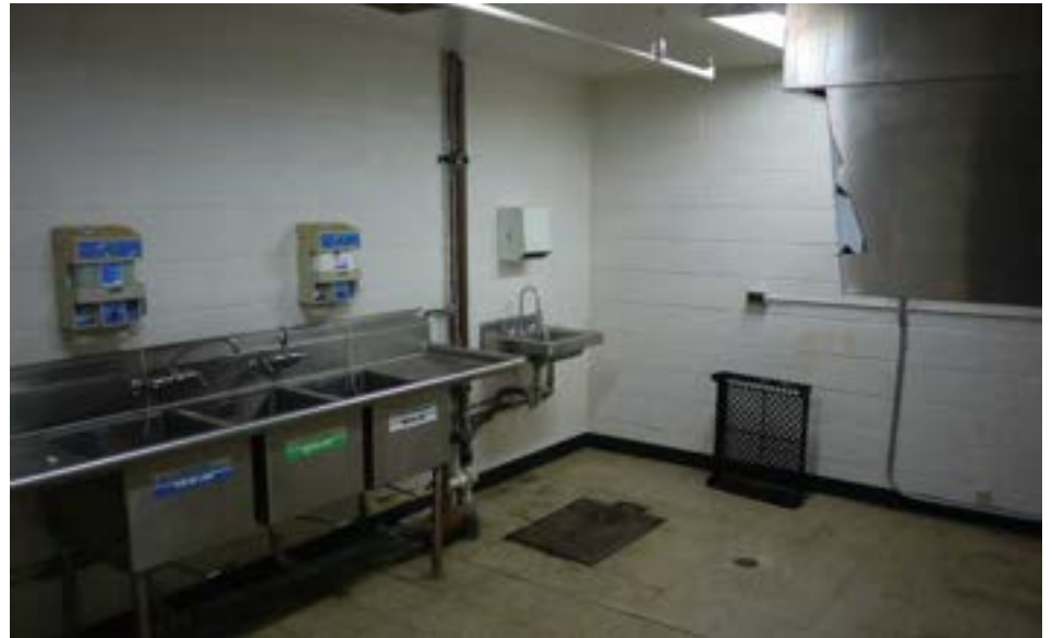
A storage room was converted into a small kitchen with commercial sinks and vent hood. The kitchen is adjacent to the multipurpose room.
