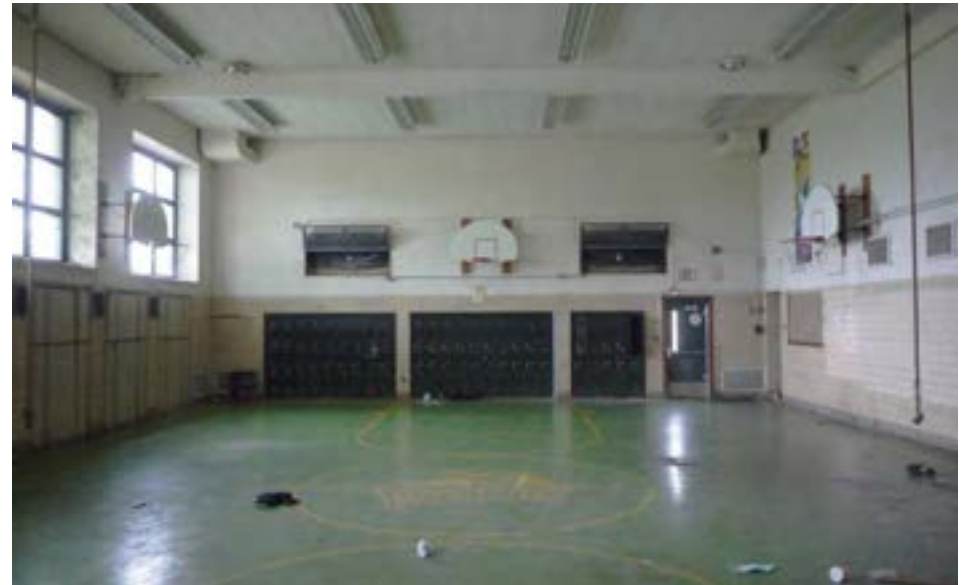
The combination gym/cafeteria is in excellent condition and features a vinyl floor.
