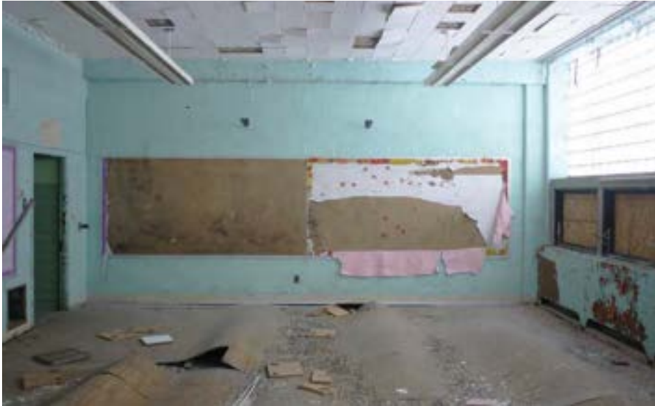
A typical classroom with simple painted CMU walls, large glass block windows over operable lites, and wood floors. Wood floors are
