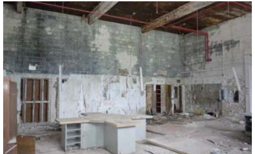
The original gym in the 1940s unit was converted into a science or art room, presumably after the larger gym was added in 1992. There is evidence that the entire upper half of the space was concealed behind a massive drop ceiling (now gone).
