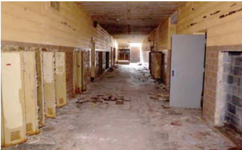
The 1954 unit's corridors are double-loaded and windowless. Pictured above is the first floor main corridor. Corridors are finished with glazed block around the lockers, and painted CMU above.
