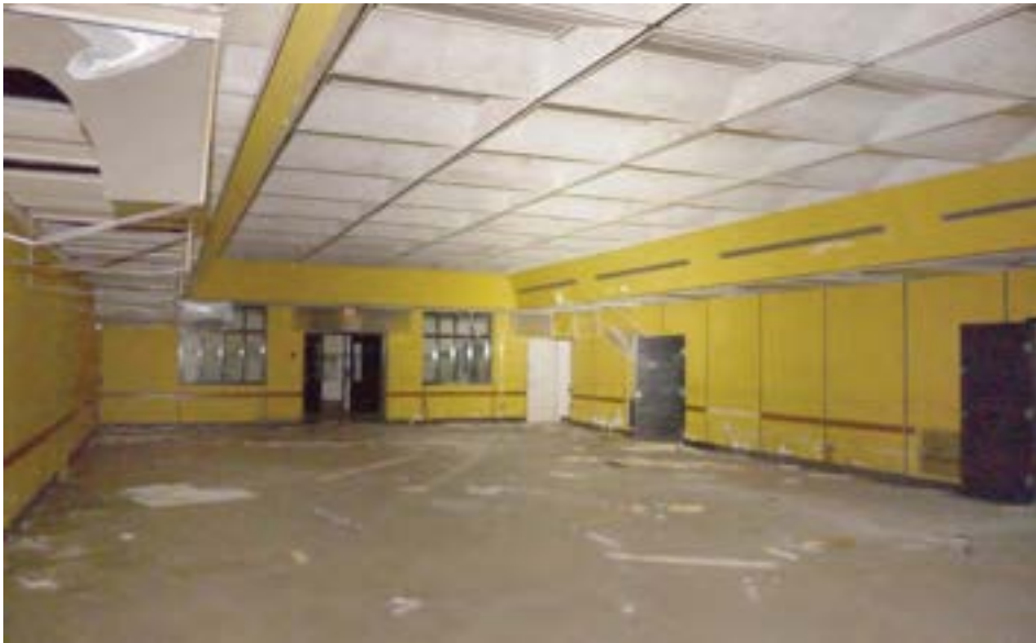
The southwestern courtyard was given a roof and converted into a large, windowless cafeteria.
