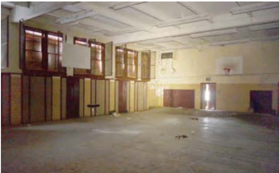
The gymnasium/cafeteria is in good condition, though the floors have begun to bow.
