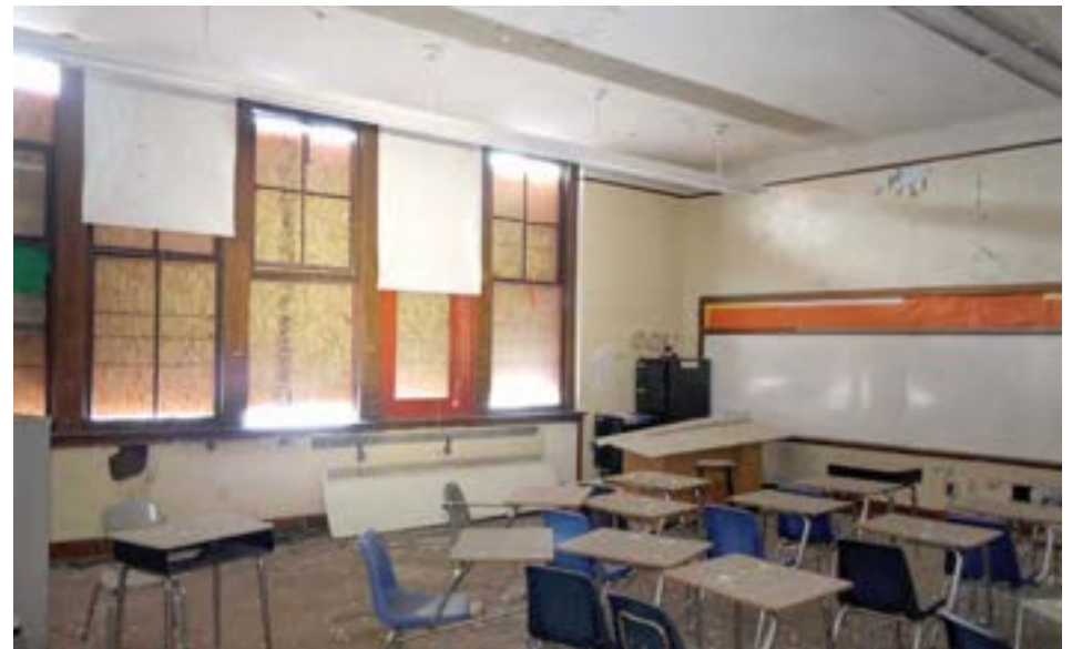
A typical classroom with intact windows and furniture. Higginbotham has been largely spared from looting, vandalism, and scrapping. Many of the original windows are still intact, and interior finishes are in generally good condition.
