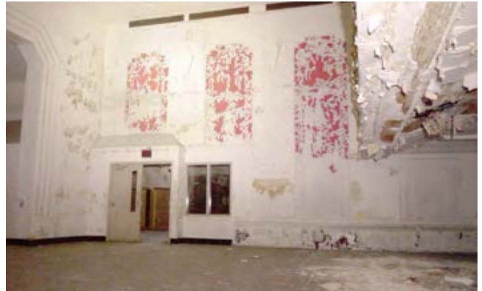
The auditorium is located in the core of the building and lacks windows for natural light. The auditorium has a tall stage and a balcony, suggesting a grand original space. However, the balcony has been walled off and converted to offices, and raised stage is gone.
