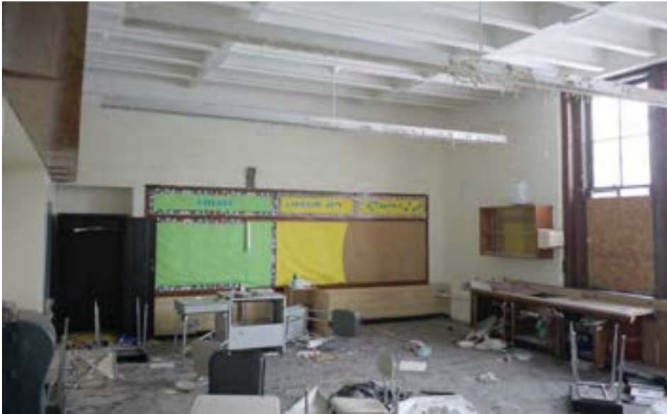
A 1940s era classroom featuring high ceiling with visible cast concrete structure left exposed. Walls are simple painted CMU, in good condition.
