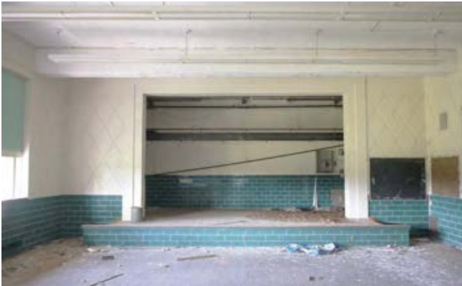
The small auditorium is finished with painted concrete and glazed block like the rest of the school, but features blocks with a decorative diamond pattern instead of plain CMU.
