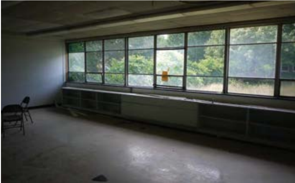
A typical 1961 classroom features wall-to-wall operable aluminum windows. Many of the glass lites have been replaced with plexiglass. Although these windows are in serviceable condition, full replacement with efficient windows is recommended rather than repairing.
