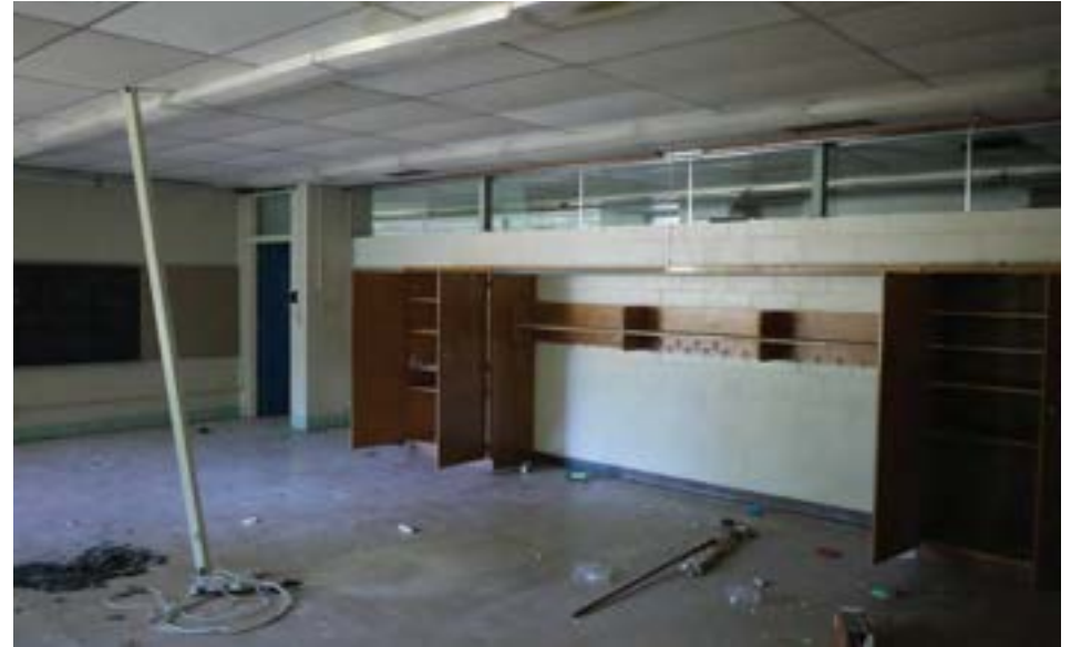
Typical 1961 classroom featuring wood cabinets and coat hanging area, and clerestory window to hallway, allowing natural light. Finishes are simple with painted CMU walls, vinyl tile flooring, and acoustic drop ceiling.
