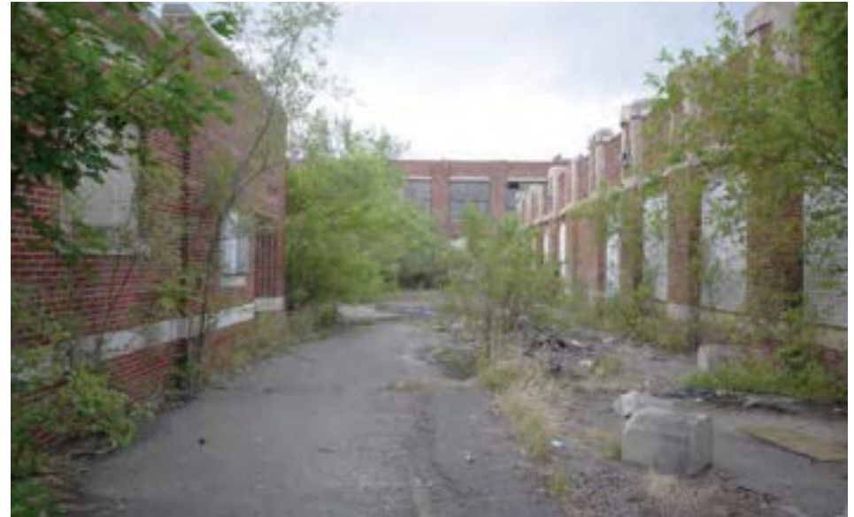
The northwest courtyard formed by the 1955 wings. The gym, pool, and locker room complex is to the left, and has courtyard access. A specialty classroom and workshop wing is to the right, while the original school building is in the background.
