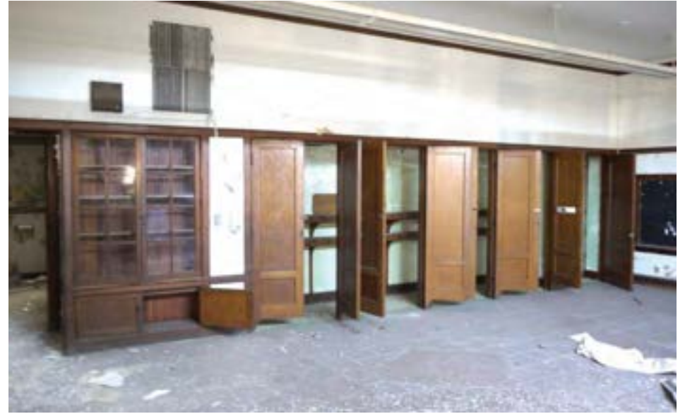
Wooden cabinetry and coat closets in classrooms in the original north unit. These coat closets allowed students to store belongings in the classrooms instead of in hallway lockers. Newer classrooms lack this feature, with metal lockers were incorporated into the hallway design instead.
