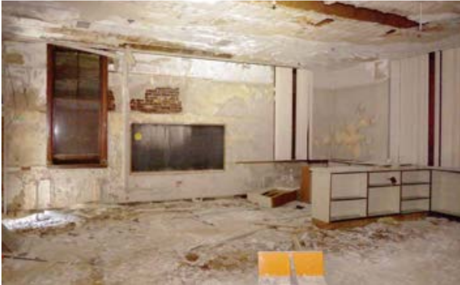
Historic floorplans show that the 1922 addition contained a small auditorium and stage on the second floor. The space, shown above, was converted into a large classroom or possibly library, and no features from the original auditorium remain.
