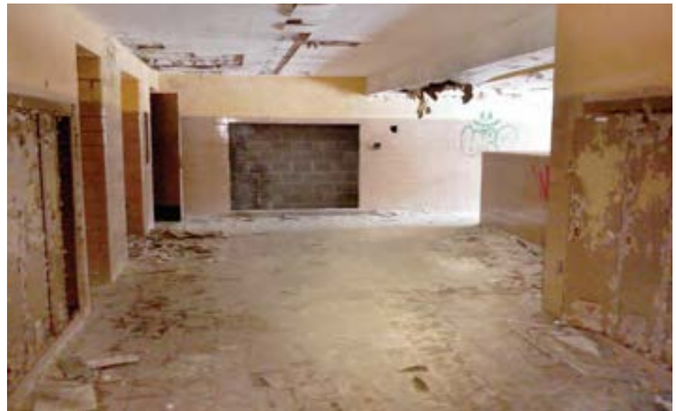
The north landing of the 1954 unit is unusually spacious and receives ample natural light from a large window in the stairwell (to right of frame).
