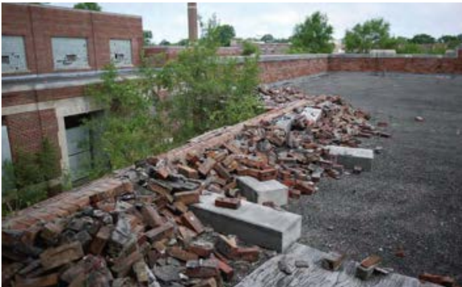
Scrapers have damaged the roof and parapet in multiple locations, leading to widespread water damage inside the building. This image shows a damaged parapet on the northeast wing of the original unit.
