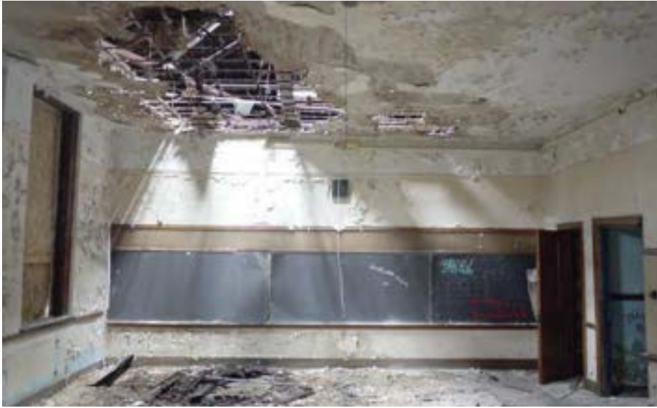
Roof failure visible in a second-story classroom on the south wing. Large openings in the wooden roof deck allow water to infiltrate the wing from top to bottom.
