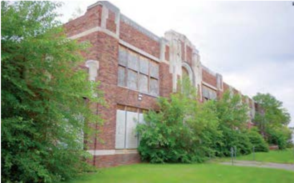
West elevation of the original school building looking south. The 1-story 1955 addition is just visible to the left of the frame, obscured by bushes.
