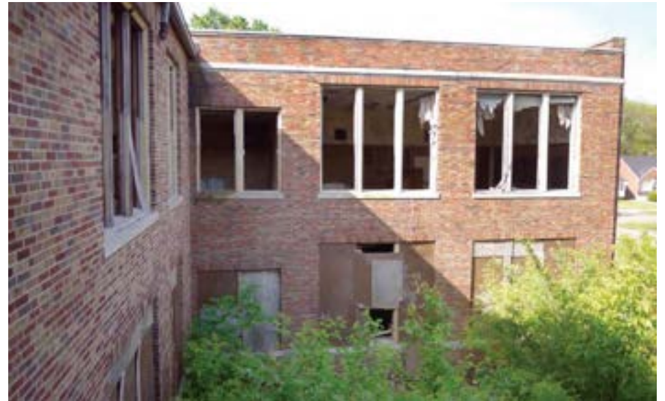
The rear (west) courtyard viewed from a second story classroom. Unlike many other U-shaped schools where the rear courtyard is paved and primarily for allowing light, this courtyard is grassy and has some small trees. However, there is no direct courtyard access from the building.
