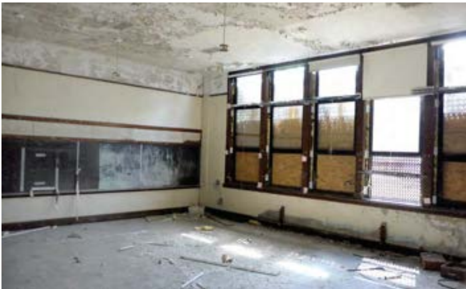
This classroom shows the original window configuration (though the original assemblies have been replaced with modern metal frames). The plaster and wood finishes shown here are typical, though in better quality than many other classrooms that have been damaged by water infiltration.
