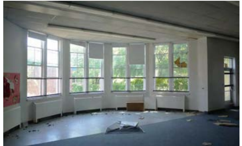
The 1925 kindergarten features a large bay window, typical of historic kindergartens. The windows and floors were recently replaced with modern materials.
