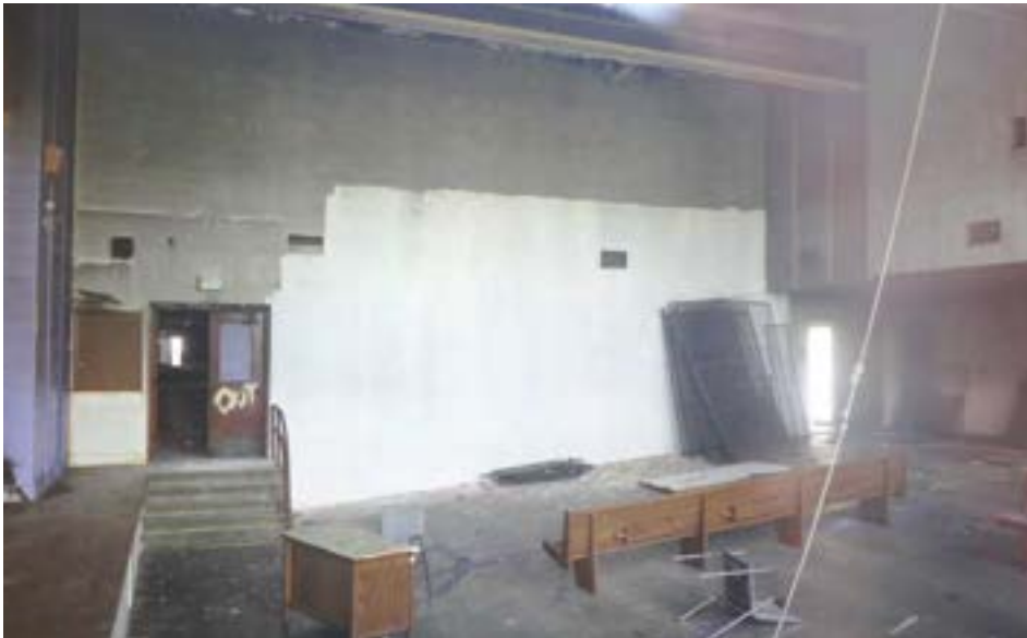
The auditorium exhibits smoke damage from a fire (location unknown, but potentially in the stage area). The white area on the wall suggests that there was either an attempt to clean the damage.
