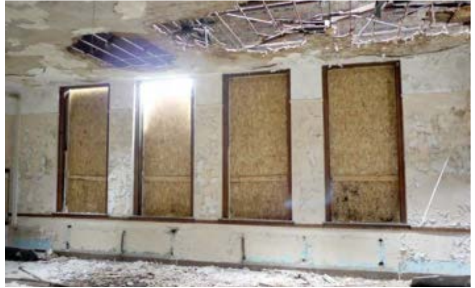
A typical classroom window configuration, featuring four separate wood-framed openings. Windows are scrapped throughout the building.
