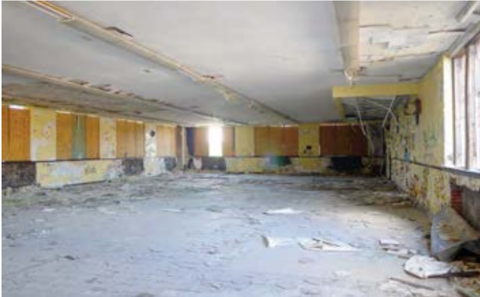
A cafeteria with a large dedicated kitchen sits on top of the two gymnasiums. With windows on all four elevations, this space would have been brightly lit and with sweeping views of the school and adjacent park.
