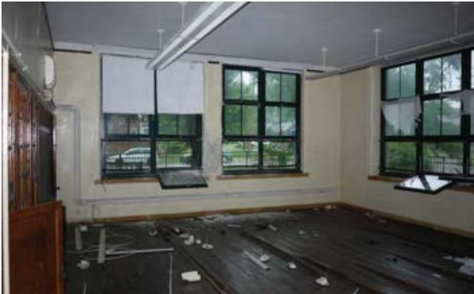
This school includes one "open window" classroom, a feature often found in 1920s era and older schools. This corner classroom features large windows on two elevations, for natural light and cross ventilation. The aluminum-frame windows are modern replacements.
