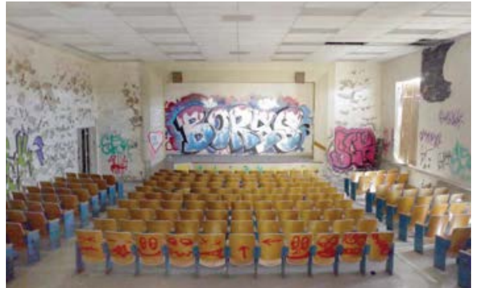
The southwest auditorium is mostly intact, though covered in graffiti. The drop ceiling conceals the original barrel vaulted ceiling more than 21' high. There is a 'twin' auditorium at the northwest corner that was divided into two classrooms; however, the stage, vaulted ceiling, and projection box remain.
