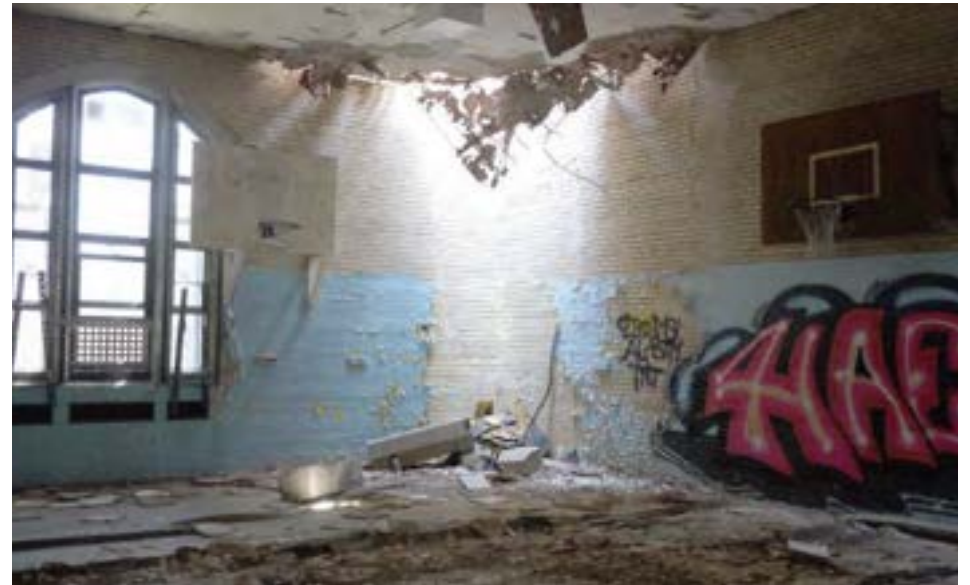
Hole in gymnasium roof caused by falling coping stone.
