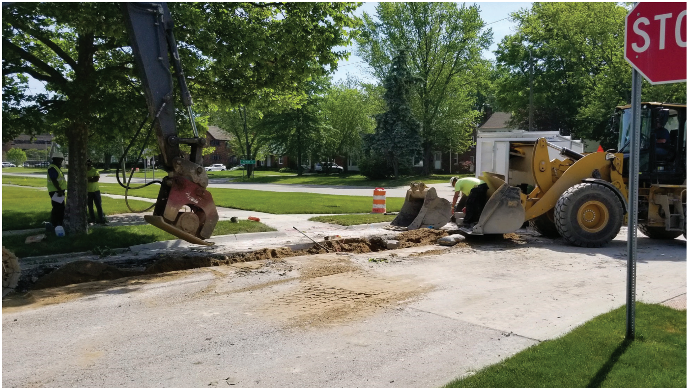
A DWSD contractor installs a new water main in Cornerstone Village, a neighborhood on Detroit's eastside.
