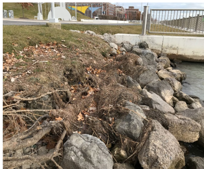
Erosion above the existing riprap shoreline
